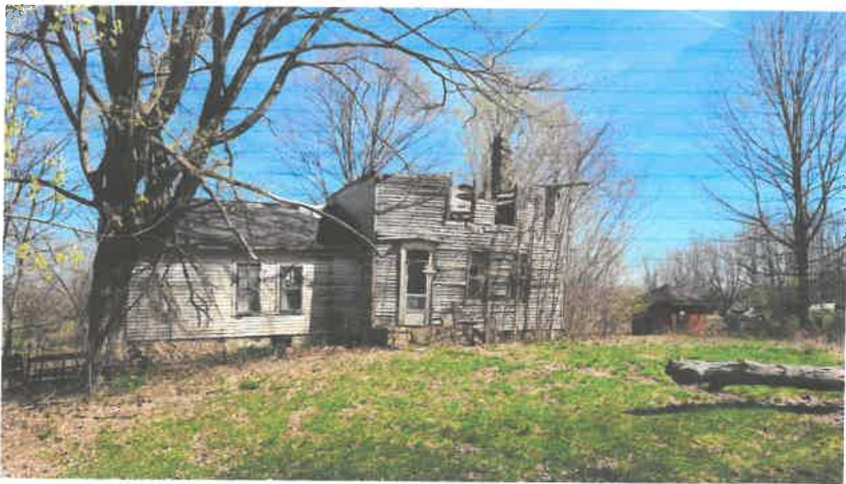
Ricky & Rhonda Deutscher Trustees, 9565 W 100 N, Michigan City, Parcel ID 460528400001000046 (abandoned since at least 2010, roof collapsed in 2021)
